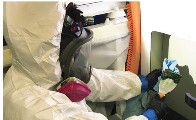
Routine mold inspection and quick removal is crucial to maintain a healthy environment.
